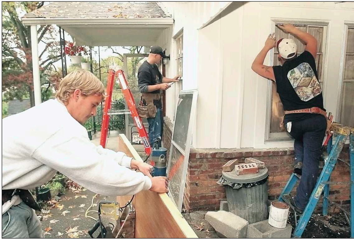
A crew from J.W. Wallace Construction Co. works to weatherize the home of Etolia Littlejohn in East Knoxville. A.J. Byers, left, routes out for the hinge on her new door while Lewis Robinson, center, and Bob Baker, right, trim away old caulking around the windows before resealing them.
